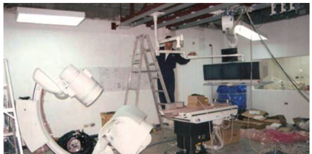
Packaging and installation of the X-ray equipment donated by the Boston Children's Hospital to UNICAR.
