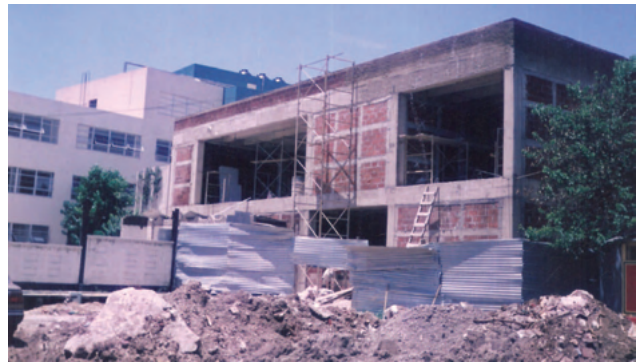
Module under construction to locate the Boston X-Ray equipment. Behind is Roosevelt Hospital.
