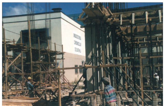
New construction, in front of the old building of the National Unit of Cardiovascular Surgery
