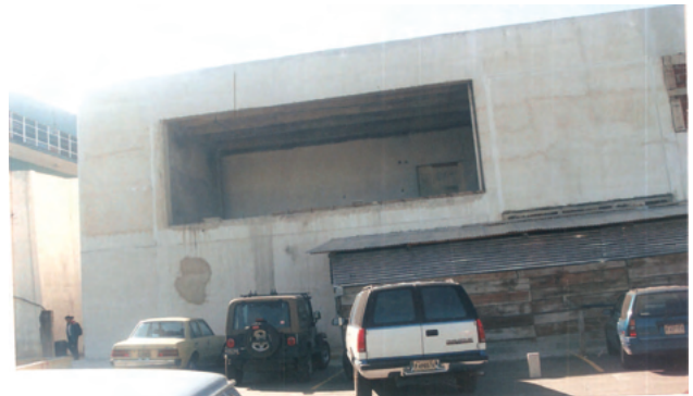
Module built in the area donated by the Roosevelt Hospital where the X-ray equipment donated by Boston will be located, which was stored in a temporary sheet metal hut for two years, to protect it from the environment.
